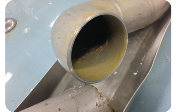
Biofilm in CIP System Pipe
