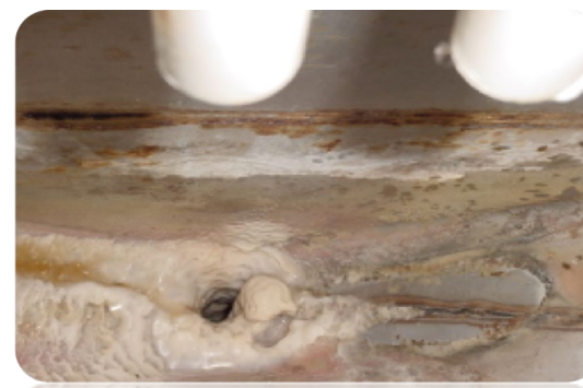
Biofilm on Bottom of Tanks
