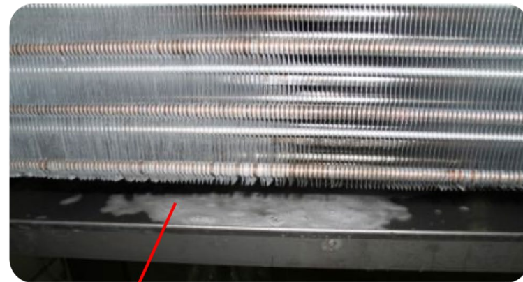
Slimy water and Biofilm in and on the surfaces of the Cooling Unit Drip Pan
