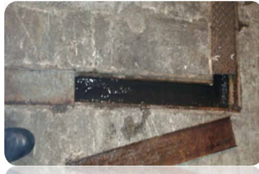
Biofilm in Drain Trench
